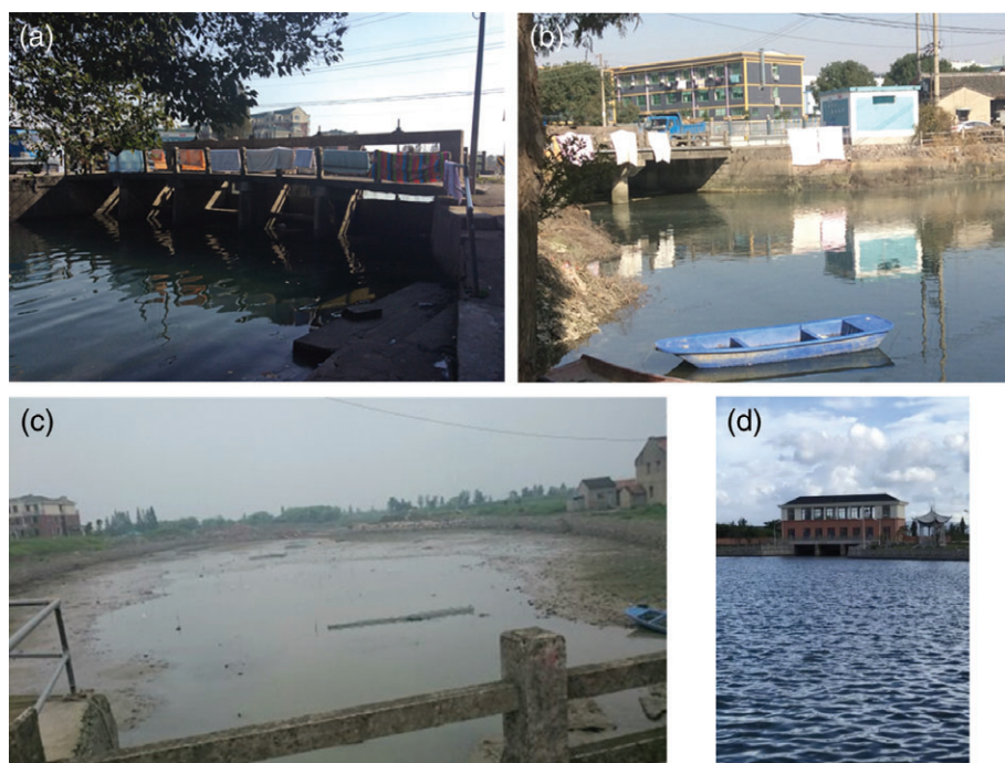
FIGURE 4 Preparation of a water gate renovation between the Nantang and Fenghua Rivers at Wujingqi at urban fringe of Ningbo. (a) The old Wujingqi from Nantang River side and (b) from Fenghua River side prior to commencement of the work in December 2014. (c) Channel connecting the Nantang and Fenghua Rivers in (b) emptied during construction in August 2015. (d) The completed new gate, photo taken in September 2017 from the position similar to (c). Photographs by the authors
