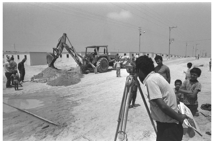
During the construction of one of Gaza’s neighbourhods, 1976. Photo by Moshe Milner, National Photography Collection.
