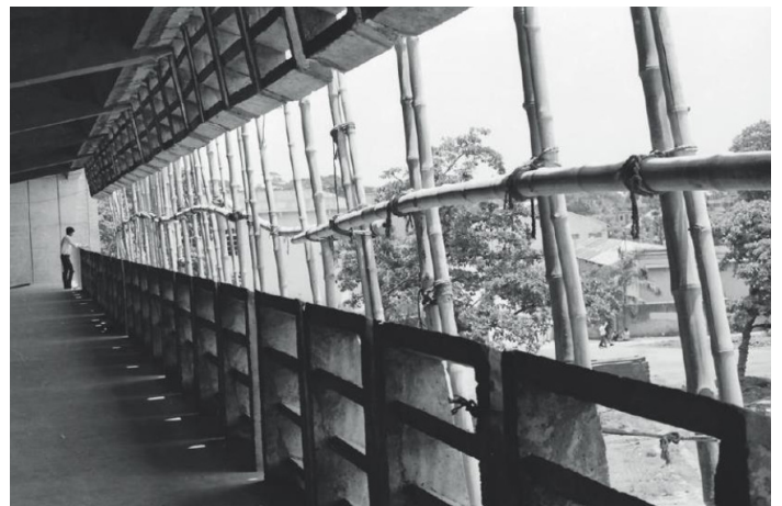
BUET Faculty of Architecture building under construction. From Islam, R. The First Faculty of Architecture in Dhaka (Dhaka: Structural Engineers, 2011).
